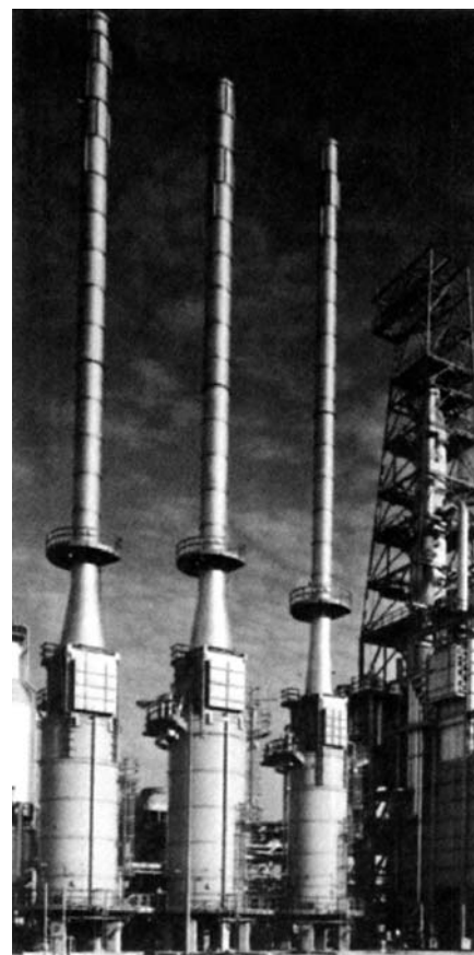
Catalytic reformer section of Marathon Oil Company Garyville Refinery showing Platformer fired heaters.
